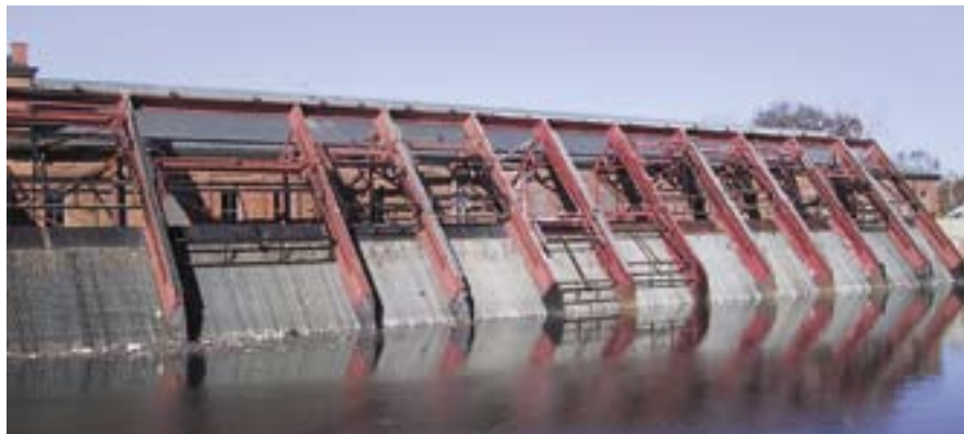
Pumping Station No. 6 is the largest of 20 stations operated by the Sewerage and Water Board of New Orleans. Because so much of the city is below sea level, storm water cannot drain by gravity and must be lifted over the levees. The steel structure in front of the station is a trash rack that keeps debris away from the pump intakes. (Photograph by Brian Hayes.)
